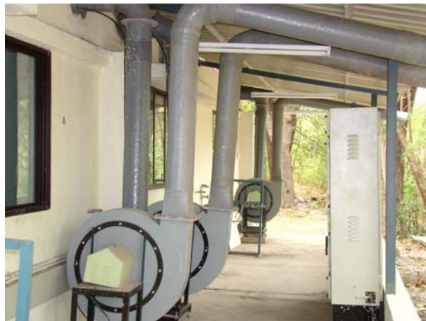
Fume Hood Blowers in Service Corridor
