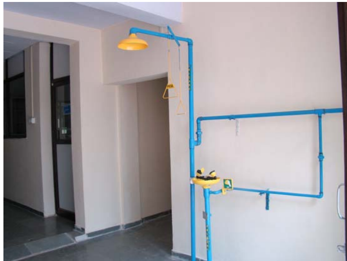
Safety shower and eye wash
