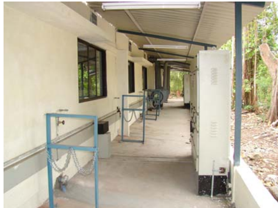
Service Corridor (for blowers, gas racks etc)
